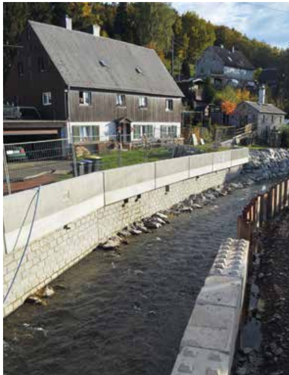
Flood protection installation in Burkhardtsdorf/Ore Mountains
